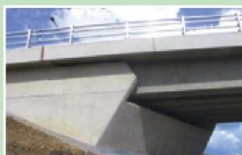
Concrete bridge abutment (on left) made with 50% Ecocem GGBS; bridge beams (right) are made with 100% OPC.
