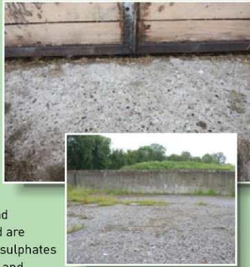
Feed channel (top), and silage pit (above) where concrete has been damaged as a result of exposure to silage effluent acids.
